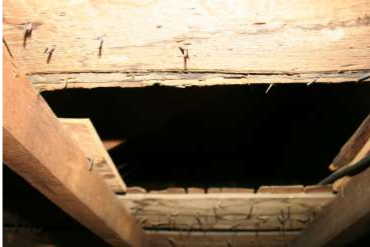
West roof slope with hole looking into portico pediment space
