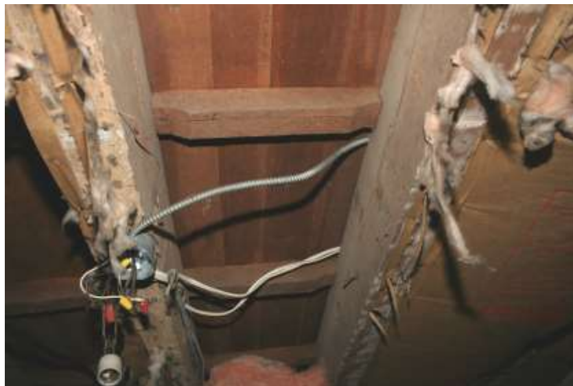
Room 001 Ceiling showing purlins notched over joists for floor boards to run east/west
