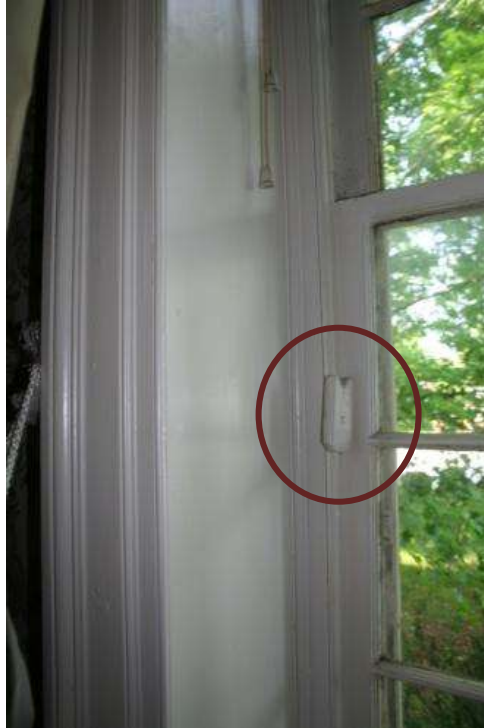
Room 102, Window 2, window sash holder (circled)
