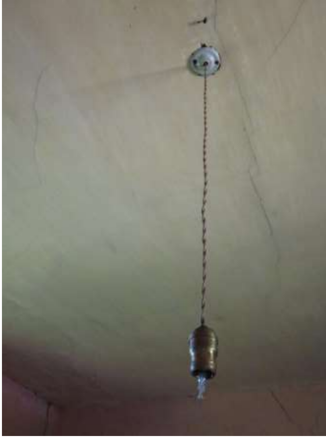
(Rm. 201) Light Fixture
