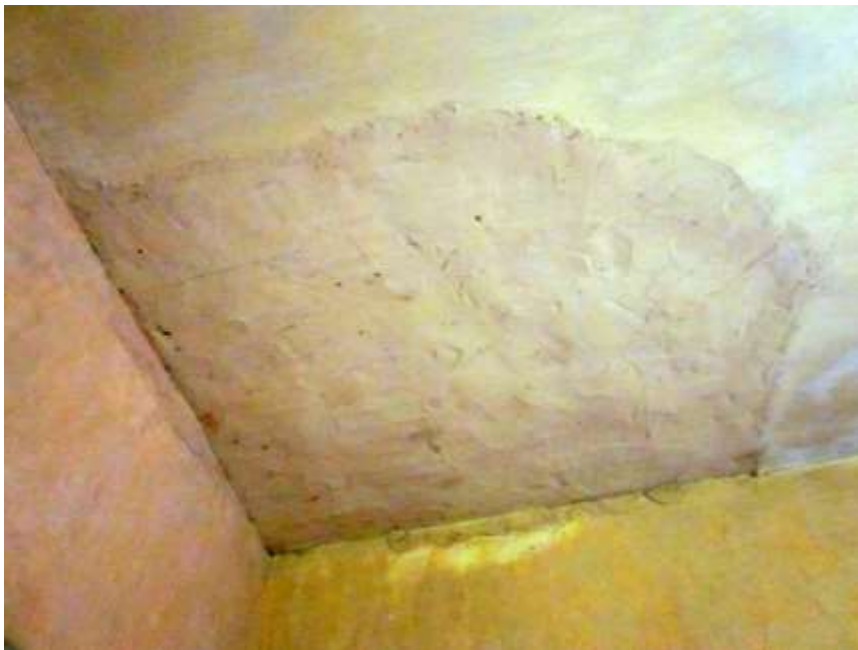
(Rm. 201) Plaster Patching on Southwest Ceiling
