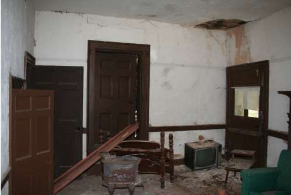
Figure X. (TM Picture ). Oakland, Room 202, south wall showing location of four doorways in room. From left, D-E-01, D-E-02, D-S-01, and D-W-01. Pictures shows the inconsistency of size and design from the east wall to the south and west walls.
