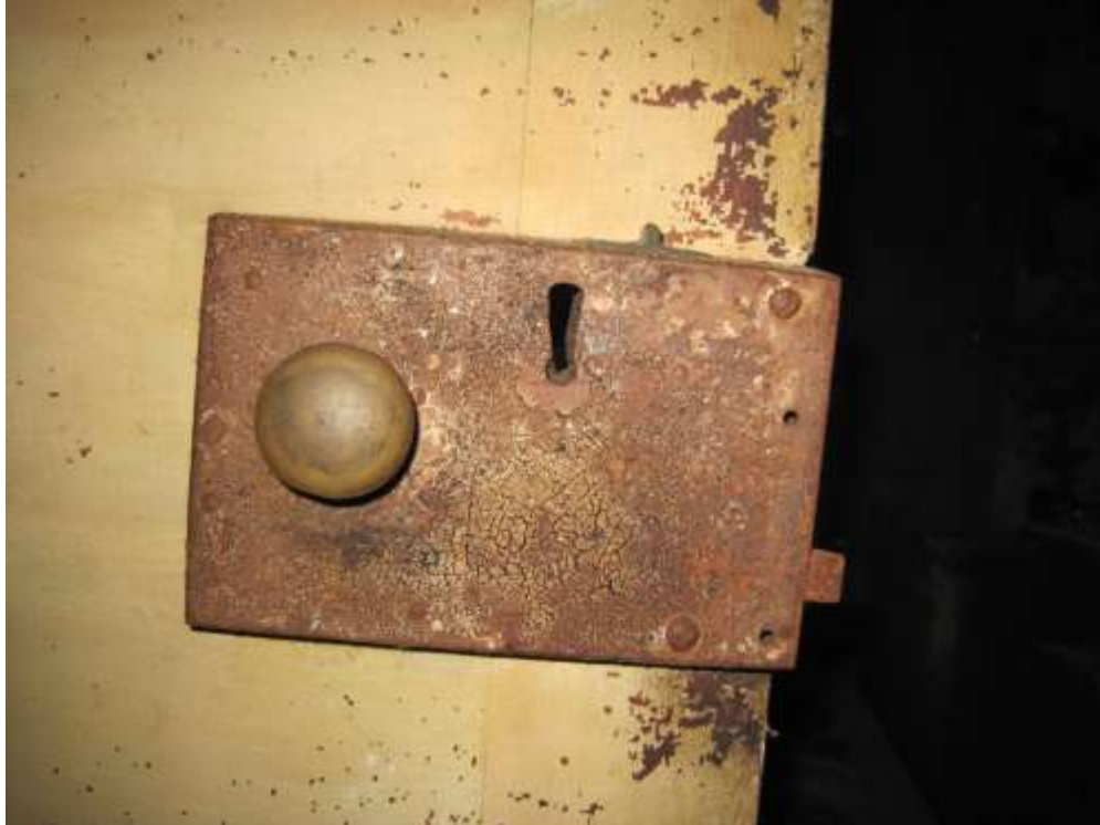
Figure X. (KF picture) Oakland, Room 202, door D-S-01 hardware. Note that lock is installed upside down.
