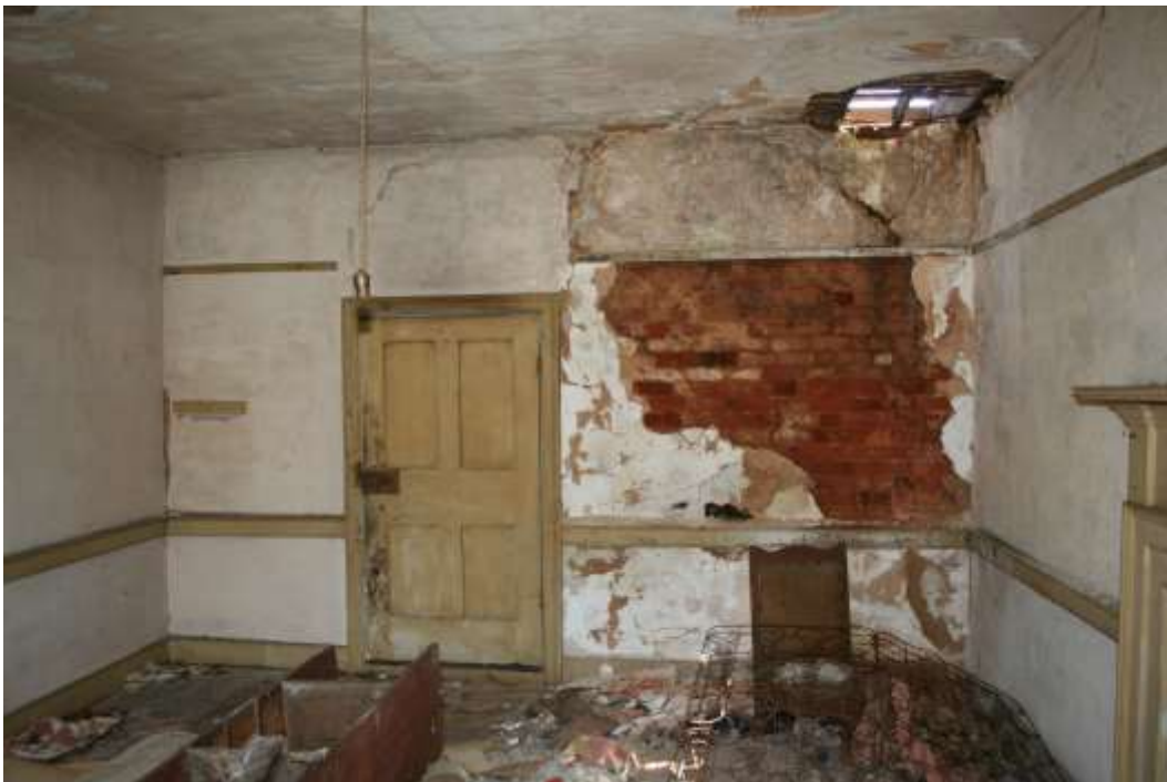
Figure X. (TM picture) Oakland, Room 202, showing door D-S-01 in south wall, exposed interior brick, and existing water damage to ceiling and wall.
