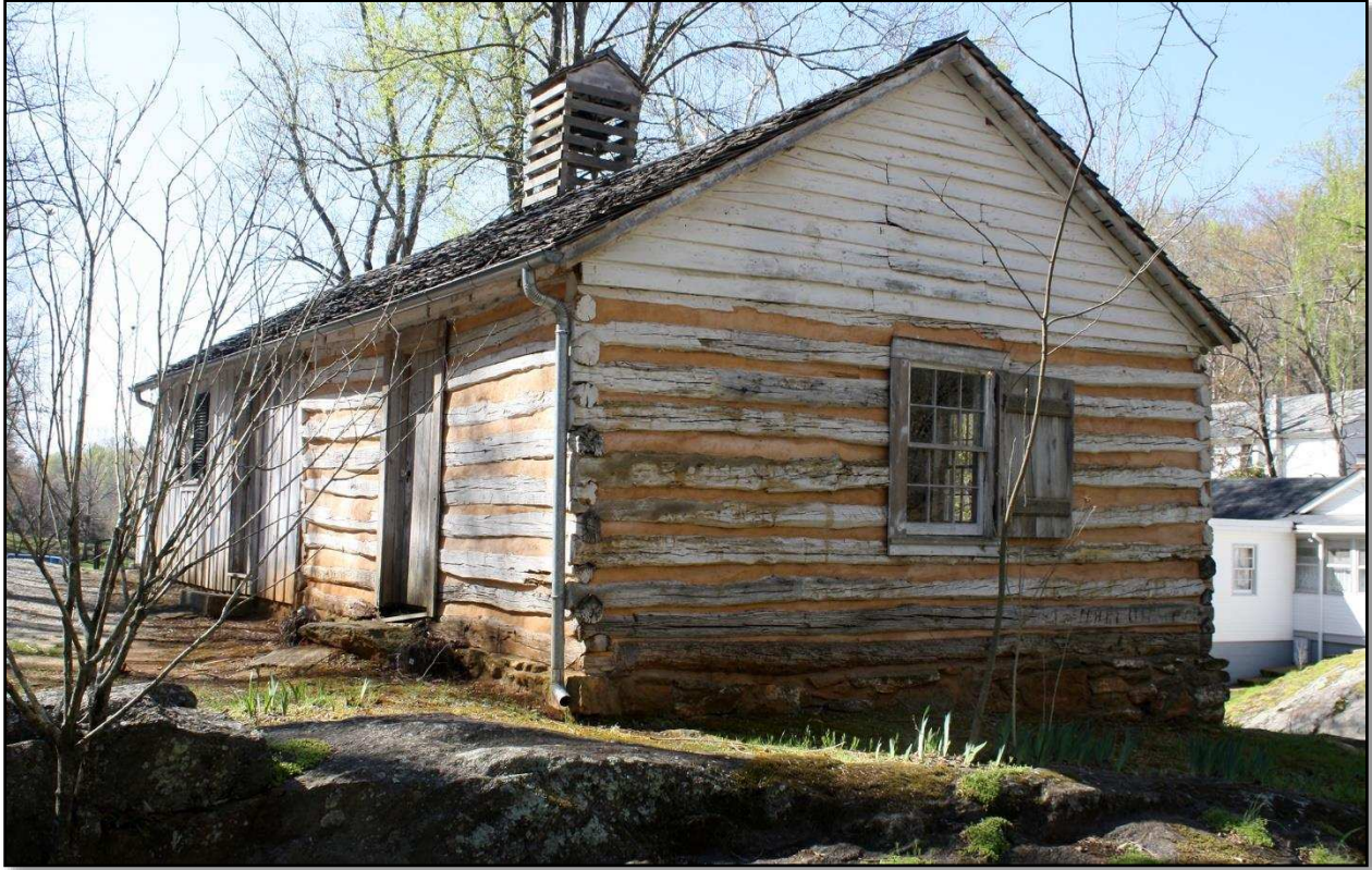
7. Side view of the restored Bear Mountain Indian Mission School, showing foundations set on bedrock. Falling Rock Creek lies behind the Mission School. Photo by the author, 2013.
