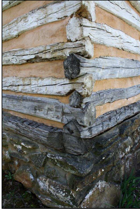
9. Detail of the V-shaped corner notching of the restored Bear Mountain Indian Mission School. Photo by the author, 2013.
