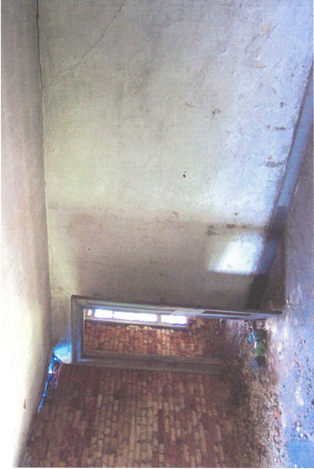
204 ↑ AREA OF GREATEST ROOF, WALL, FLOOR DAMAGE
