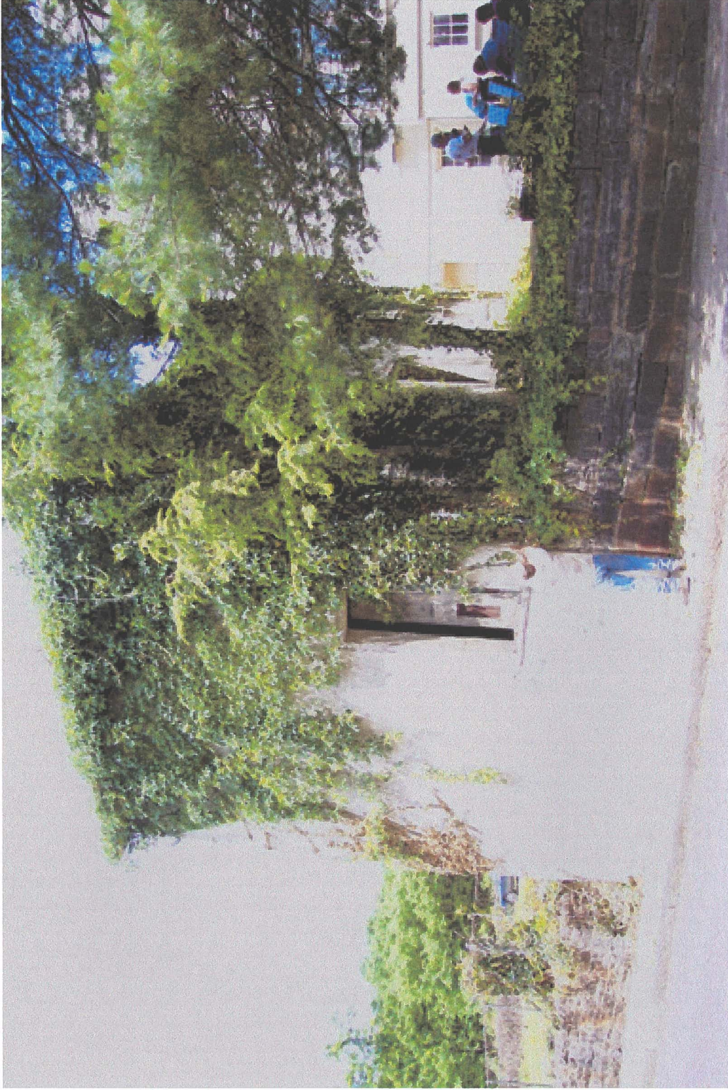
TYPICAL IVY GROWTH TO BE REMOVED AND KEPT OFF OF BUILDING
