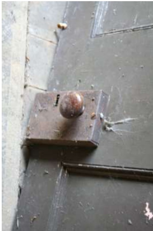
Figure 18.0- South Door Lock. Room 100
