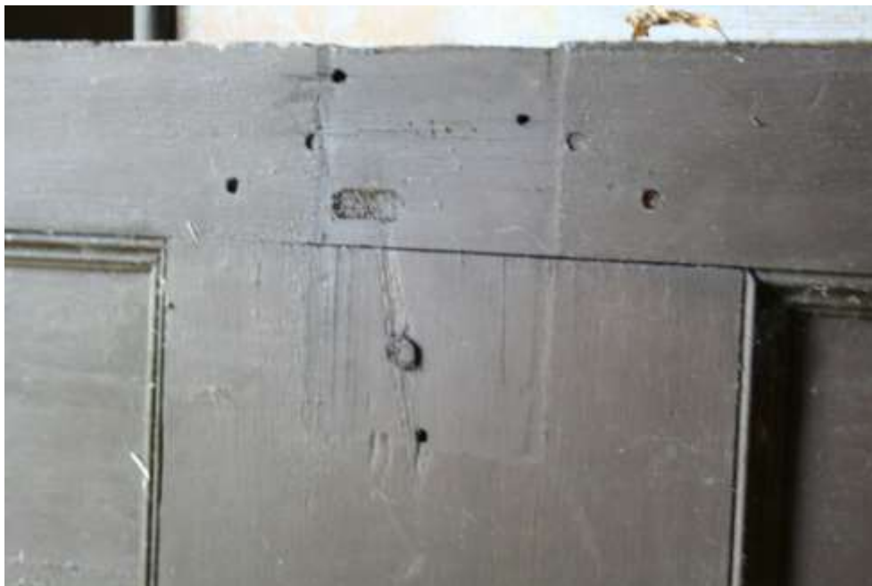
Figure 19.0- South Door Ghost Marks of Earlier Lock Placement. Room 100
