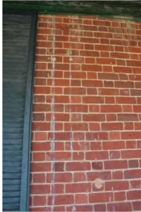
Figure 15.0- Ghost Mark from Earlier Column. North Façade
