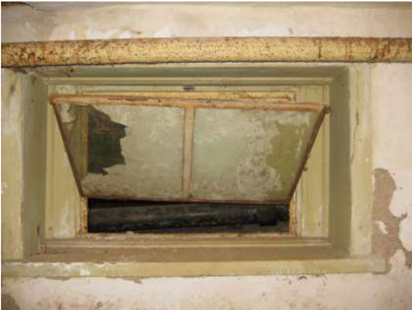
Room 002, window on east wall, K. O'Shea
