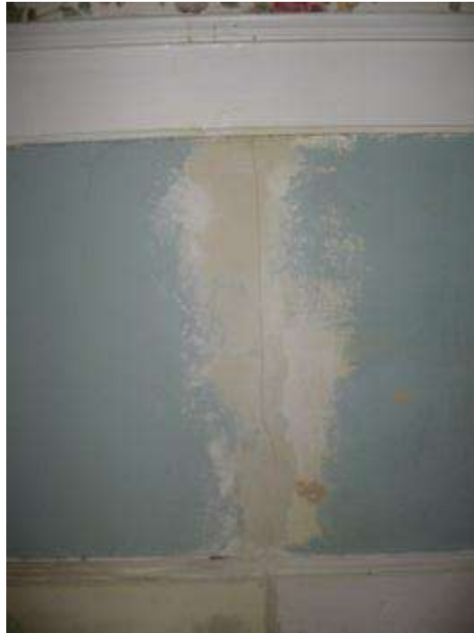
Room 102, west wall, detail of repair to plaster wall between base and surbase, K. O'Shea
