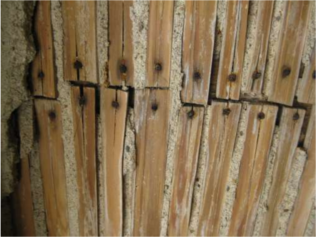
Room 002, Ceiling, K. O'Shea
